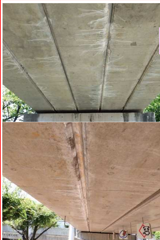
①②床版：遊離石灰
